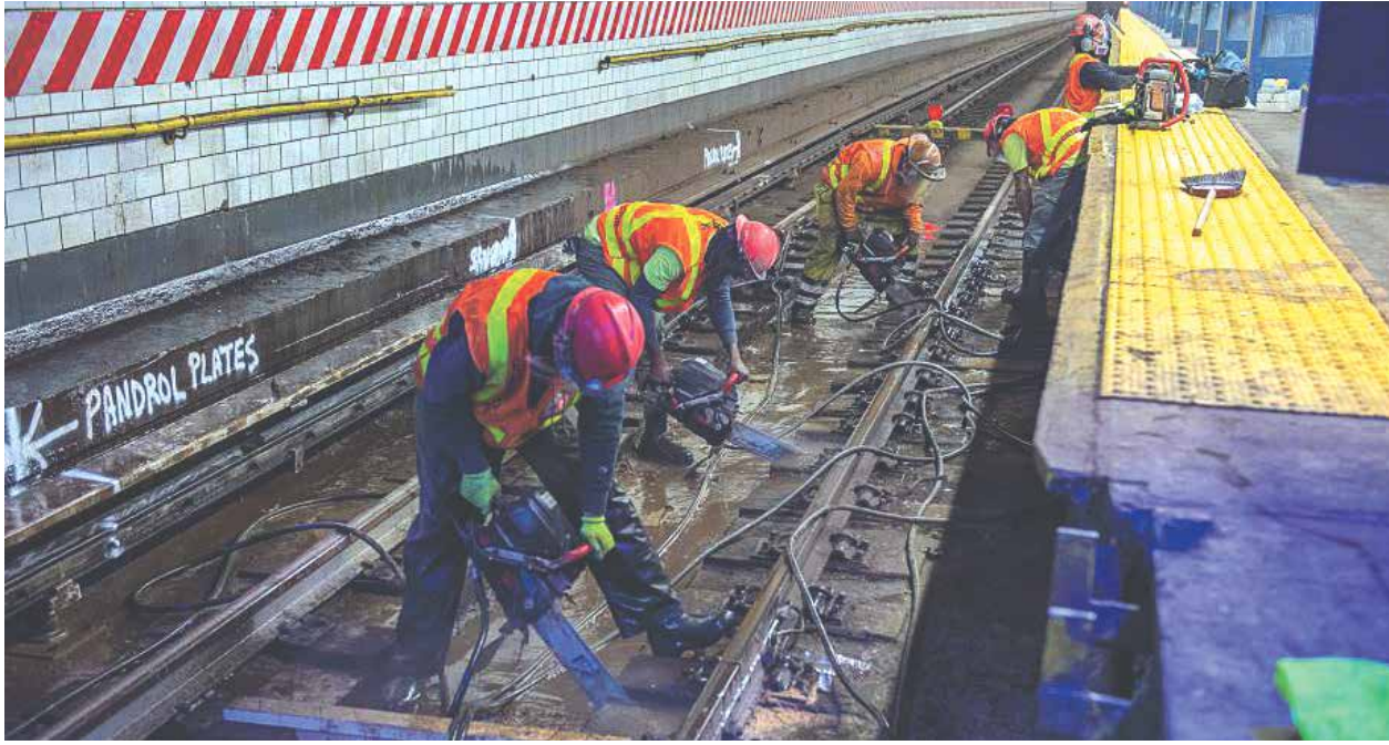
Track workers repaired damage in the Rutgers Tunnel under the East River caused by Superstorm Sandy.
